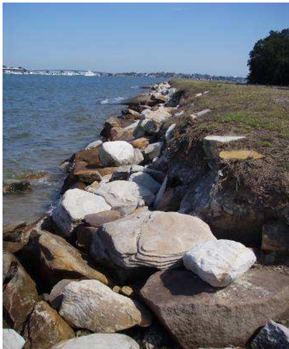
Figure 7.40 – Eroded seawall at Dover Park
