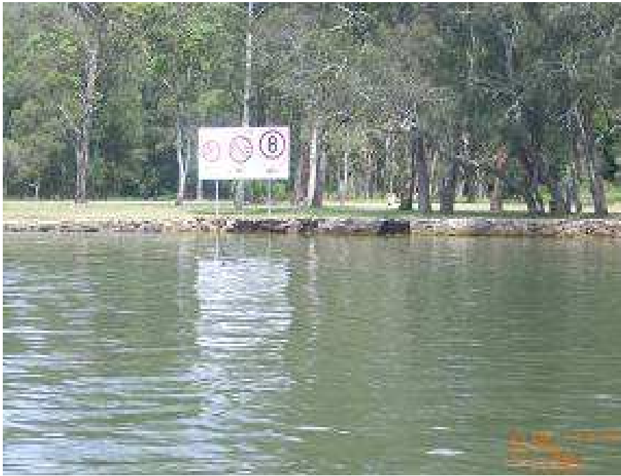
Figure 7.29 – Seawall needing light maintenance east of Picnic Point
