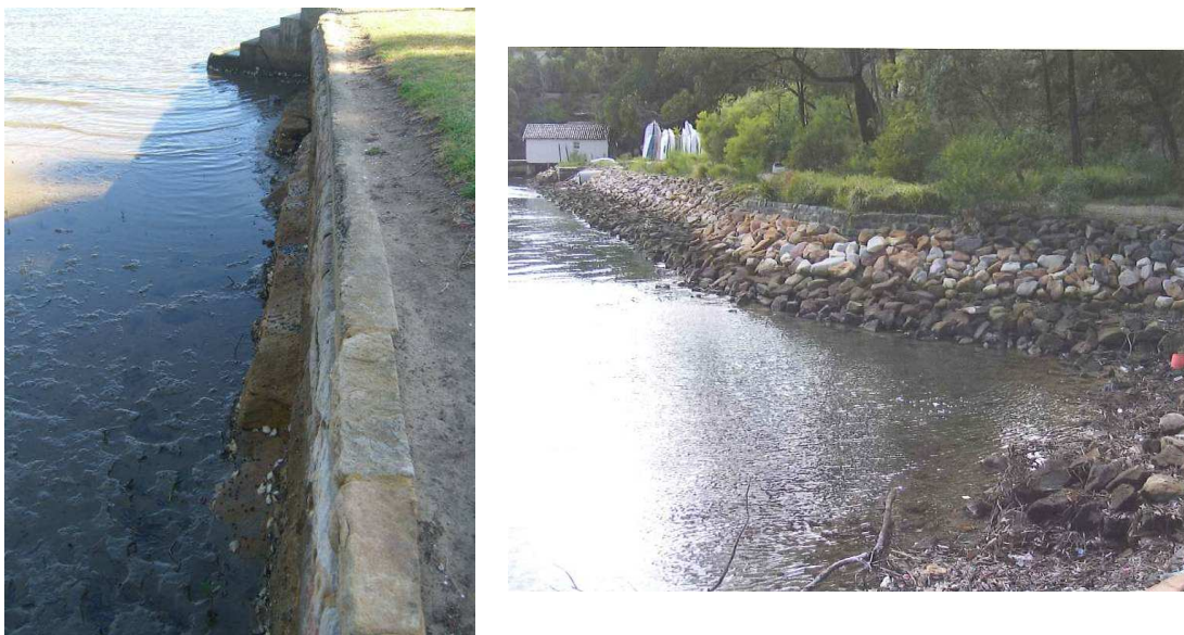
Figure 7.59 – Vertical seawall along Carss Park (left) and possible improvement from DECCW, 2009 (right)
