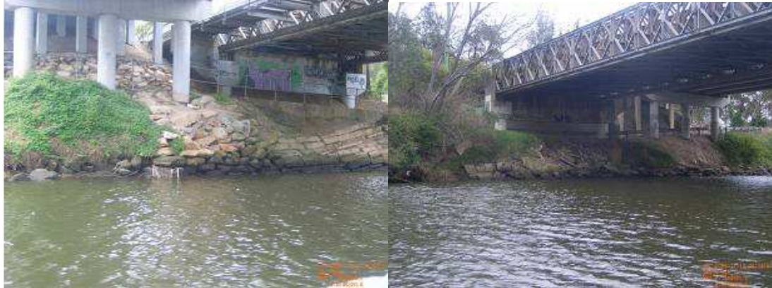
Figure 7.6 – Protections under the eastern (left) and western (right) side of Governor Macquarie Bridge
