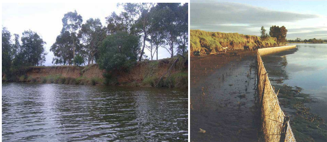
Figure 7.50 – Severe erosion on steep and height bank at South Park (left) and possible solution* from the DECCW, 2009 (right)
