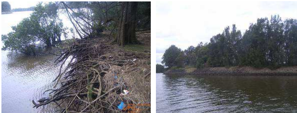
Figure 7.57 – Erosion along Wildlife Island (left) and possible solution e.g. along Daruk Island (right)
