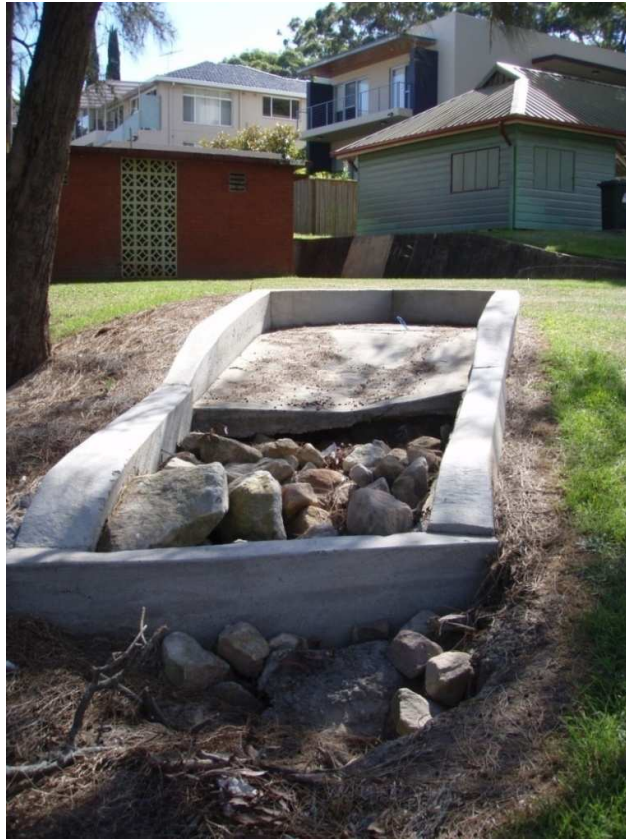
Figure 7.67 – GPT/Stormwater overflow outlet at Connells Point Reserve
