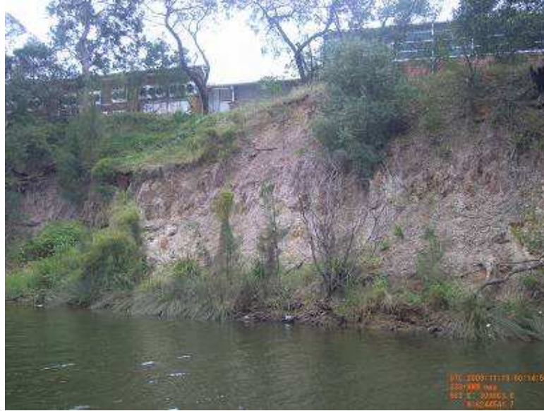
Figure 7.1 – Severe erosion between Liverpool Weir and Moore Lake
