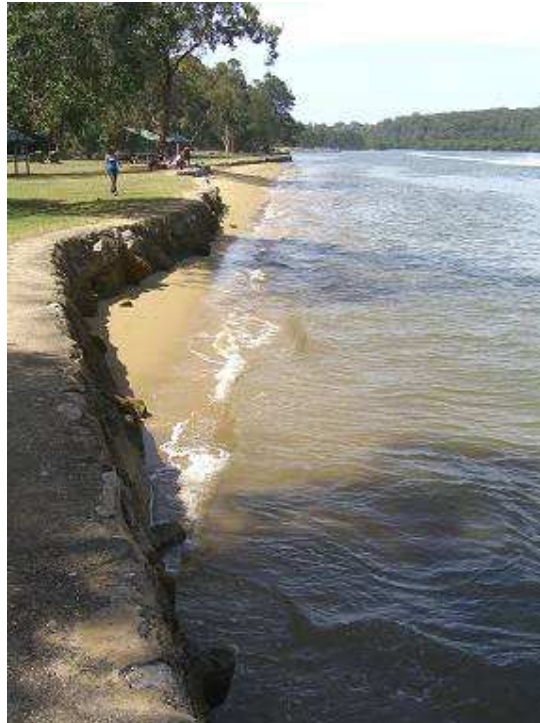
Figure 7.31 – Pocket beach along the seawall west of Georges River National Park carpark
