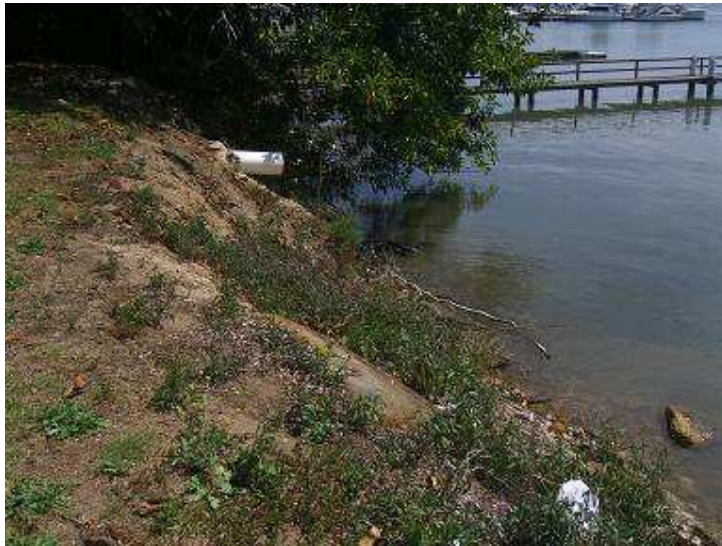
Figure 7.39 – Erosion at Dover Park West
