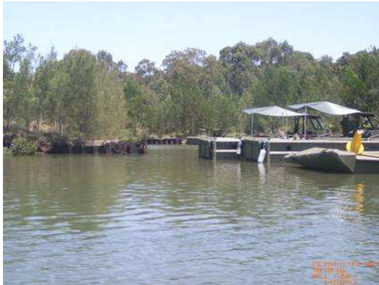
Figure 7.26 – Sheet pile protection at the military entrance upstream of Deadmans Creek mouth
