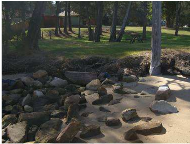
Figure 7.37 – Erosion at Connells Point Reserve
