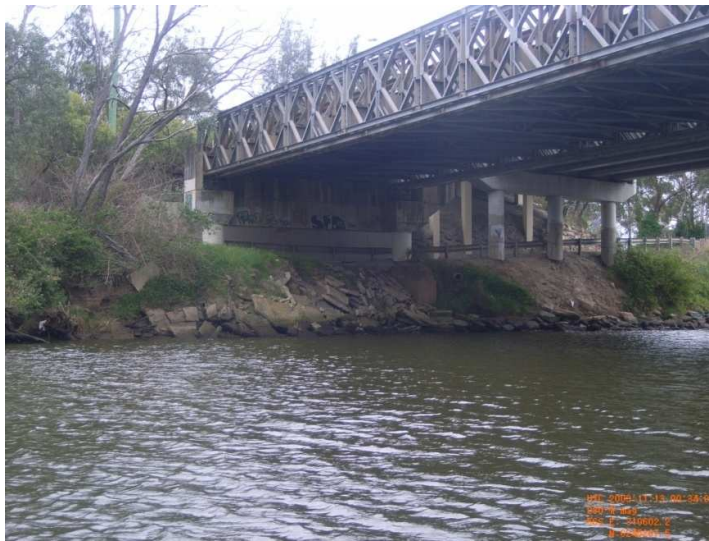
Figure 7.65 – Example of poor condition protection located under Governor Macquarie Bridge
