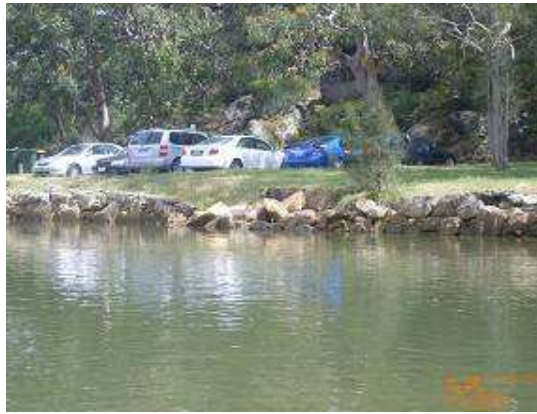
Figure 7.30 – Seawall needing light maintenance east of Anvil Rock
