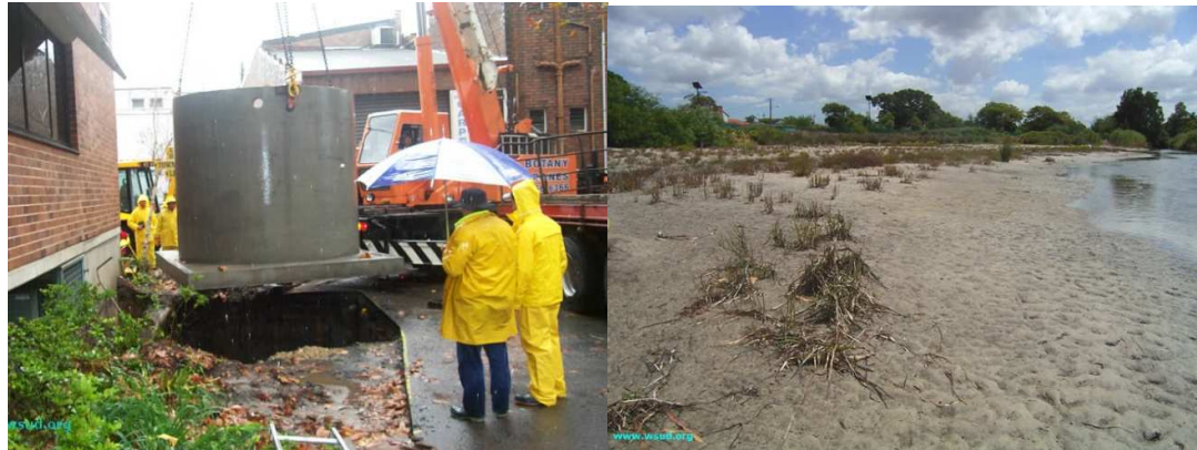
Figure 7.71 – Installation of a rainwater tank (left) and constructed wetlands (right) within Rockdale LGA
