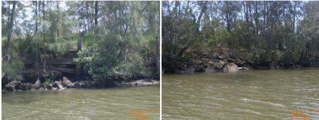
Figure 7.14 – Remnant of a timber retaining wall (left) and dumped concrete plate (right) at Hollywood Park
