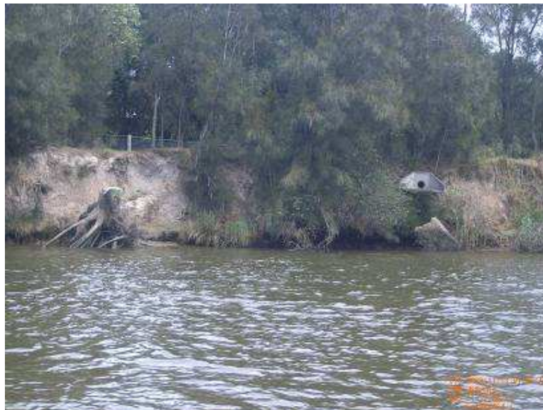
Figure 7.10 – Erosion directly south of Long Point
