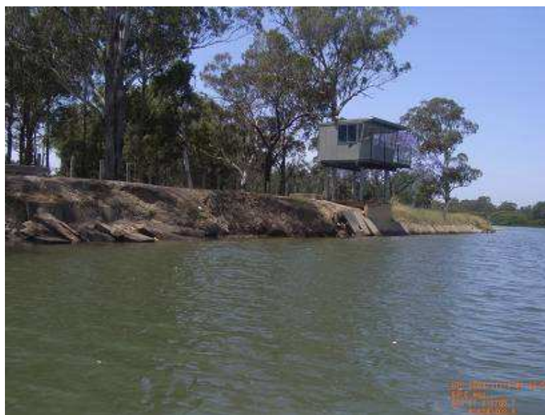
Figure 7.23 – Eroded seawall opposite Williams Creek
