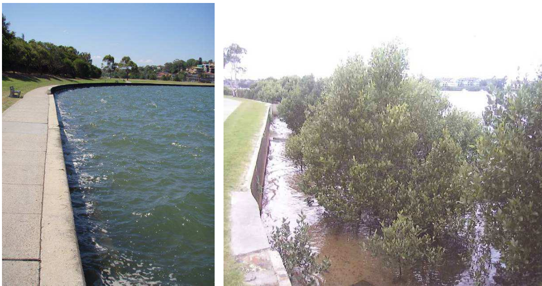
Figure 7.63 – Vertical seawall along Carss Park (left) and possible improvement from DECCW, 2009 (right)
