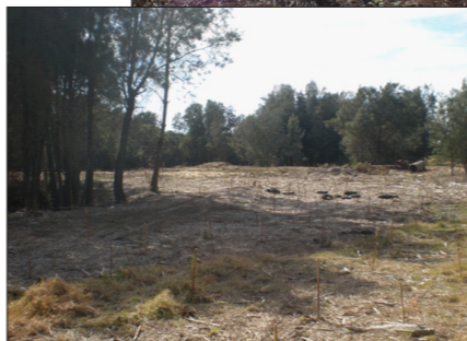
Before (top) and after photos of weed removal and revegetation works along Hassall Street, Wetherill Park. Weeds included privet, blackberry and green cestrum. Indigenous plants were sourced from Fairfield Council's Native Nursery.
