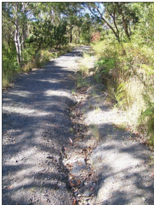
Steep access trail sheeted with asphalt scalps and shale, but with no drainage protection.
