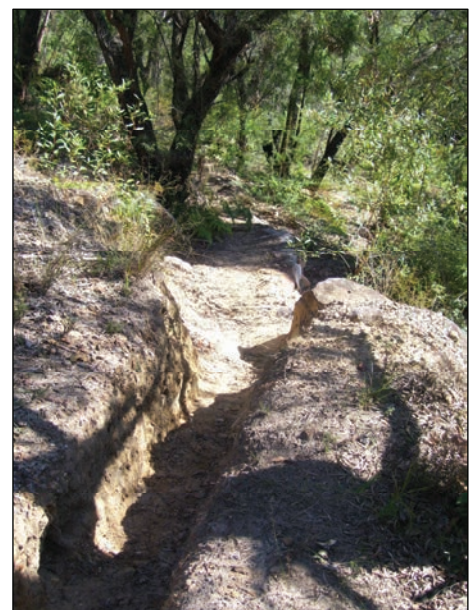
Mountain bike track cutting and erosion, east of Mill Creek at a short-cut on the fire trail network.
