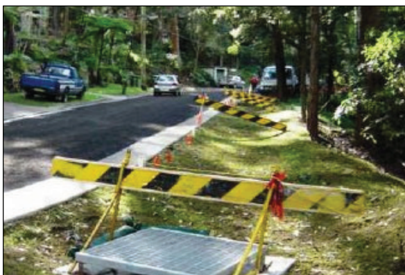
Retrofitting a vegetated (grassed) roadside drainage swale, in a similar sandstone hillside environment to the Mill Creek Catchment residential areas.
