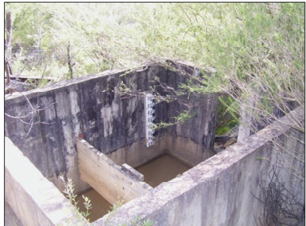
Many of the water quality devices associated with the Sandy Point Quarry are no longer operational.
