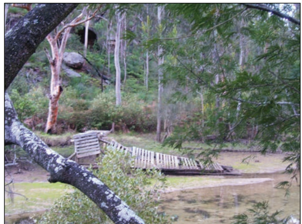
Remains of an informal bridge over Mill Creek, below Ferrier Drive.
