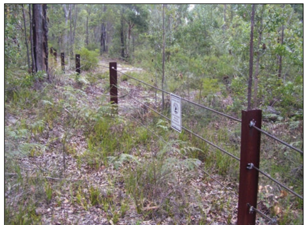
Heavy duty fencing – similar to that recently installed along the southern boundary of Georges River National Park – could be used to partition the Gandangara LALC lands to support track closures and 4WD/trailbike management.
