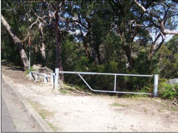
Treloar Place entry gate, low security level and repaired multiple times.
