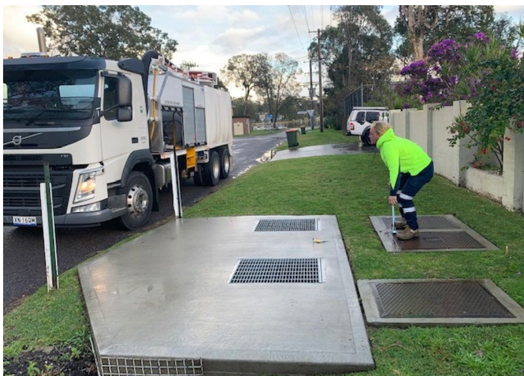
Figure 18 A number of lids require removal for operation & maintenance of GPTs and a number of lifting tool are needed – that includes for auditing too!
