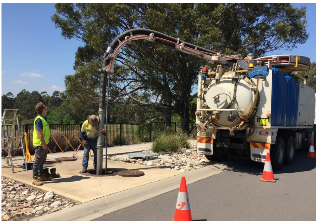
Figure 13 Example of working area around the GPT designed for safe access and operation.
