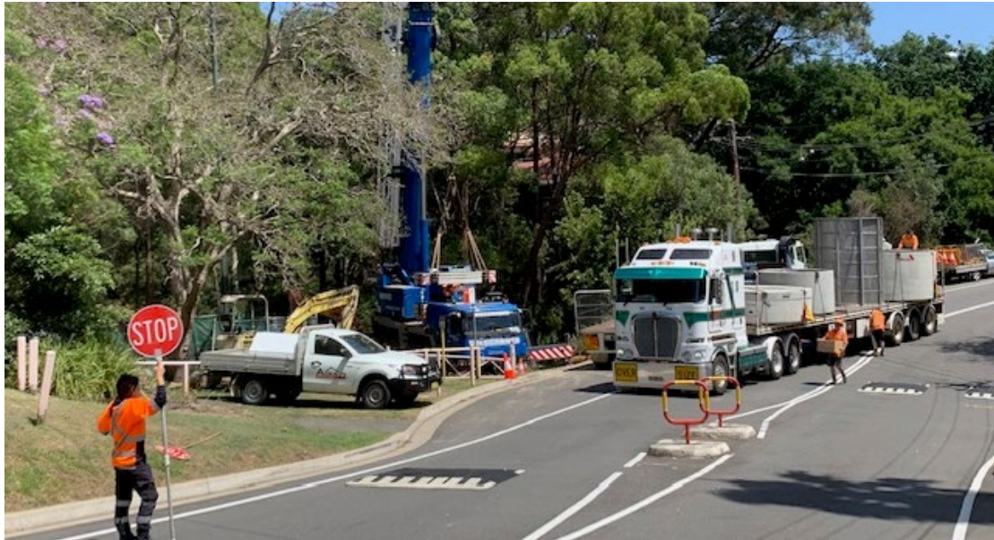
Figure 14 Delivery of the GPT to site requires careful coordination with supplier, crane operators and traffic control.
