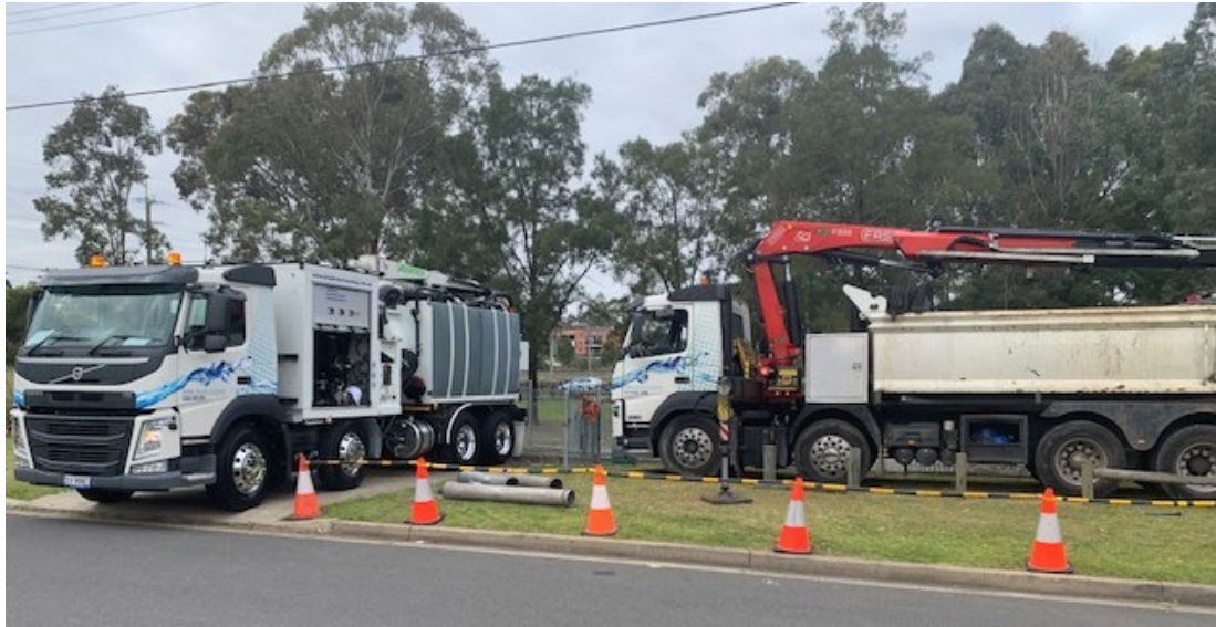
Figure 15 Cleaning large GPTs require specialist industrial cleaning plant. Seen here is a "Combo Suction Jetter Truck" and the vehicle on the right with the big red arm is the "Grab Truck".
